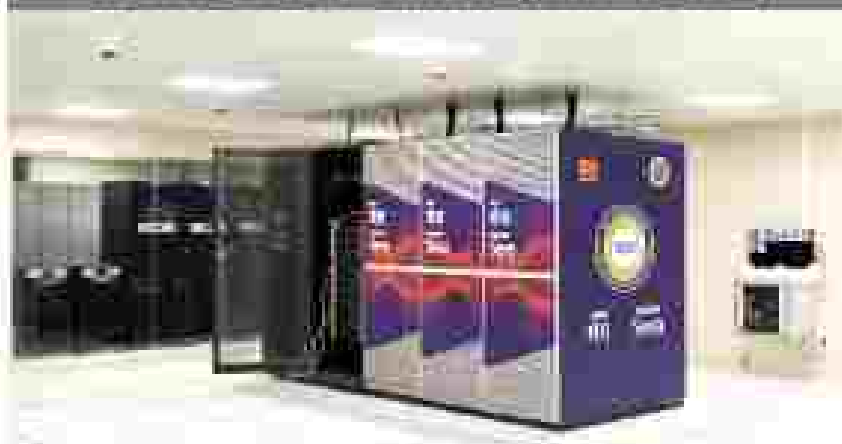
ECD TF High Performance Computational Facility
